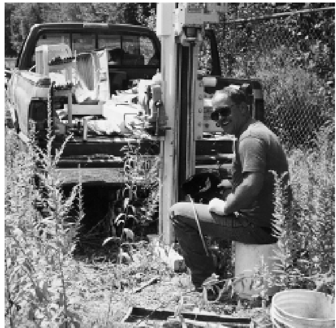
Site investigation using Geoprobe™ device for efficient determination and delineation of site contamination
