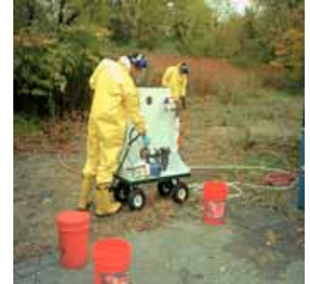
Groundwater treatment of solvents with a low pressure pump
