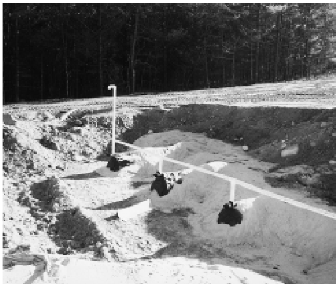
760LF PVC vent pipe for venting of leaching field
