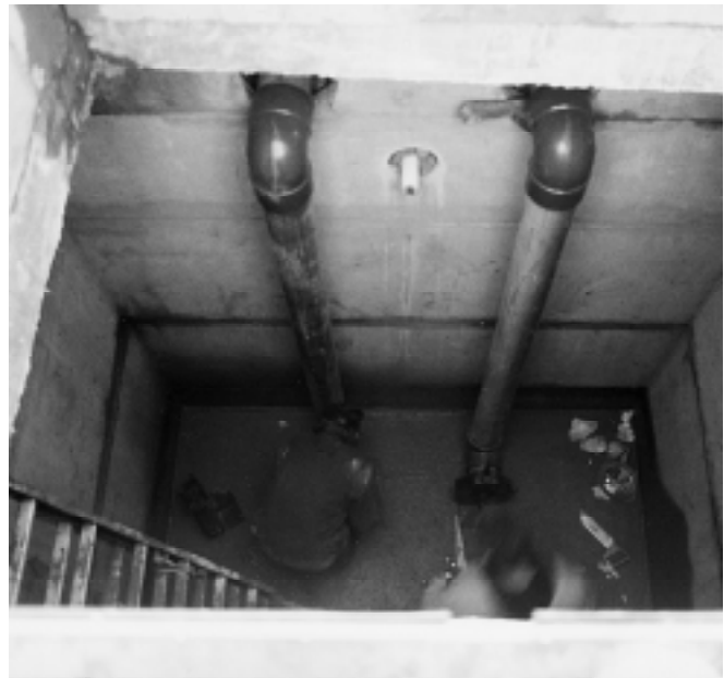
Pumping chamber with pumps, controls and alarms.
