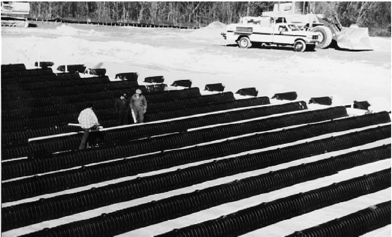
Septic system's leaching field with Coltec infiltration chambers
