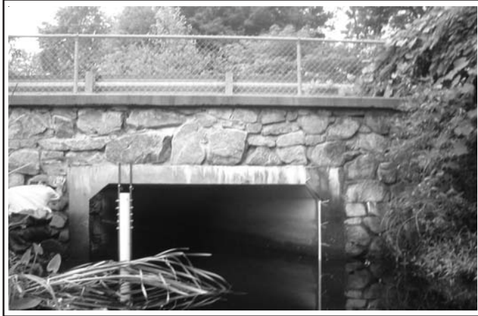
Monitoring station at Aaron River culvert at Doane Street
