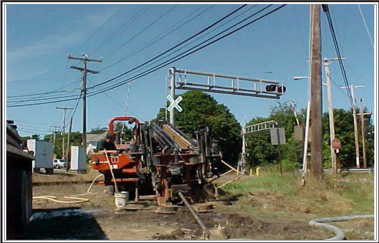
Figure 1, Horizontal Directional Drilling, in Order to Connect the Pump Chambers to the Nearby Town Sewer Manhole.
